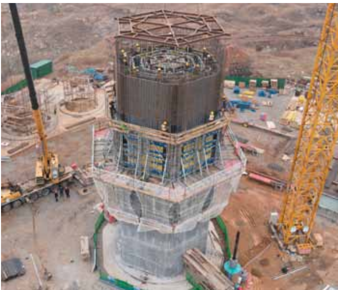
Figure 3 Lifting and Arrangement at its Final Position of the Pre-assembled Reinforcement Cage
