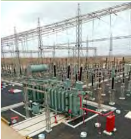
220kV Ostro Sub-Station
