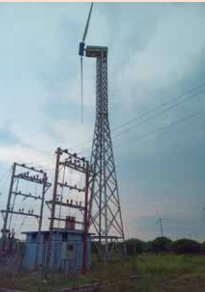
▲ Das Lagerway 250 KW turbine installed in 1995 and still running well
