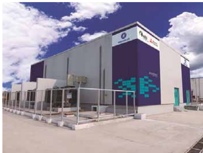
Figure 11: A 10 MW Battery Storage System in a Substation at Rohini, Delhi 9
