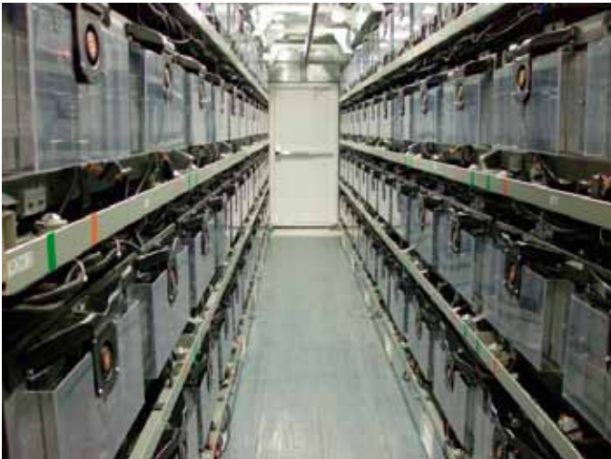
Figure 6: Lithium-ion Battery Bank for Energy Storage
