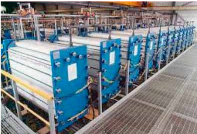
Figure 7: Flow Batteries Storage System
