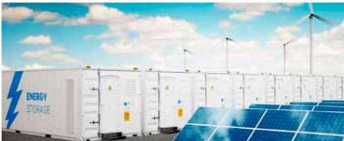
Figure 10: Solar-Wind 60 MW Hybrid Power Project with Energy Storage in Australia
