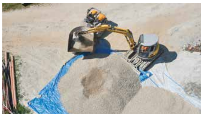
Figure 4: Gravel of Thermal Storage
