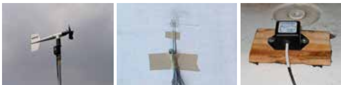
Figure 5: View of propeller anemometer, strain gauge instrumentation and tri-axial accelerometer
