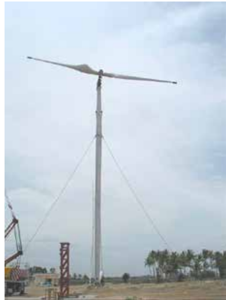
Figure 3: Field testing of 60 m tall guyed tower supporting 500 kW capacity down-wind type wind turbine
