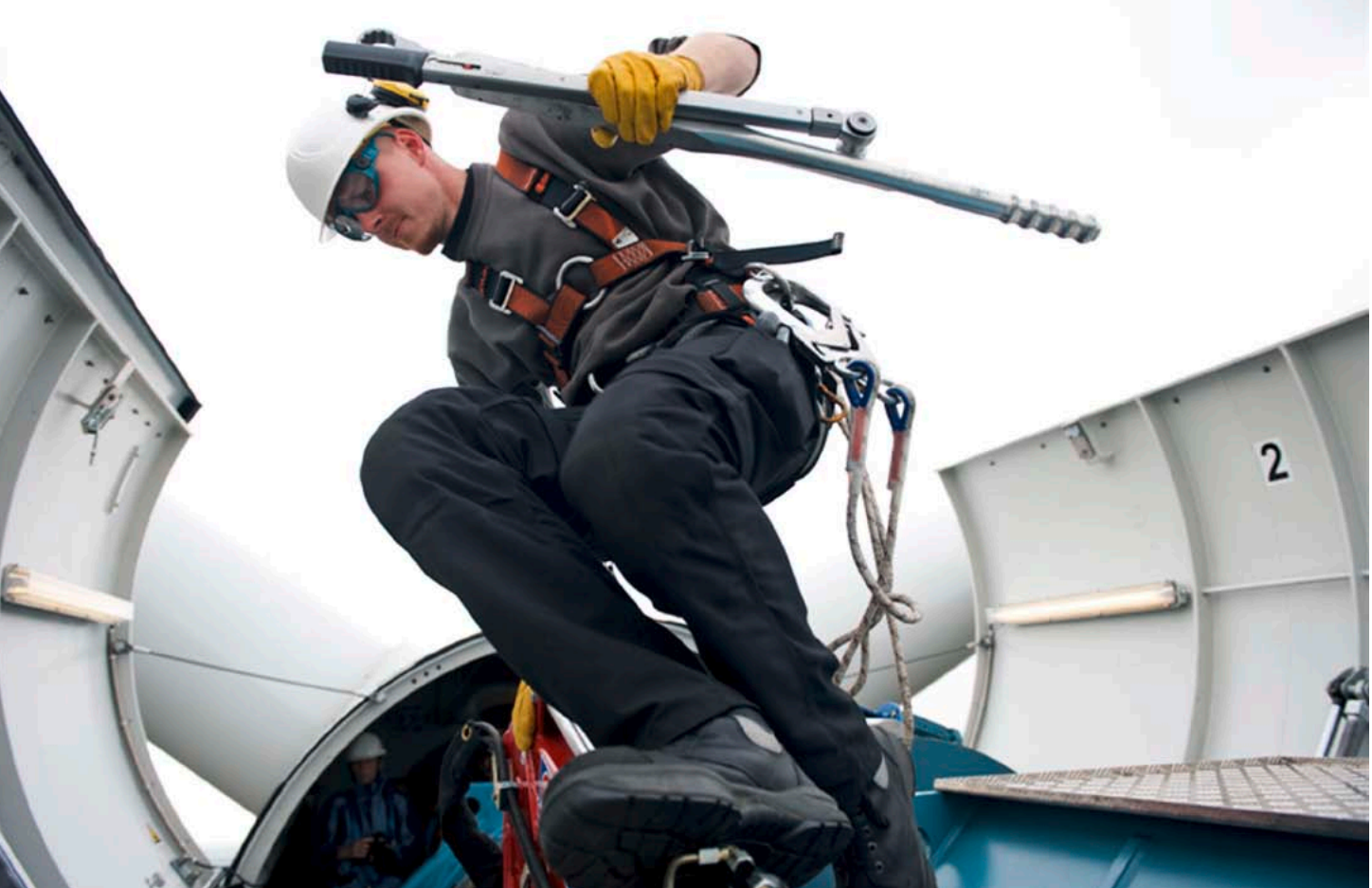
Marienkoog wind farm, Niebüll, Germany © Wind Power Works
