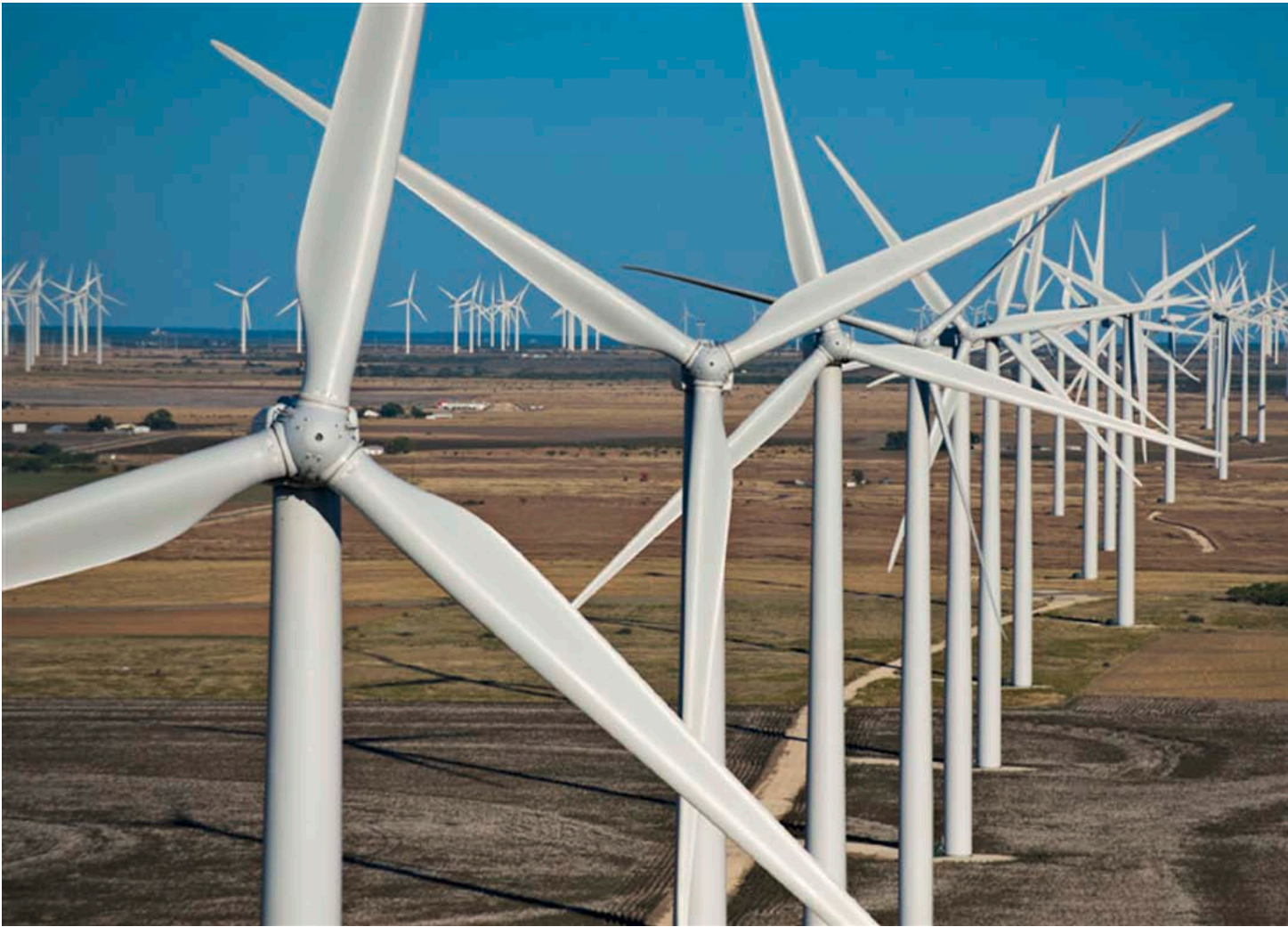
Horse Hollow wind farm, Texas, USA © Wind Power Works
