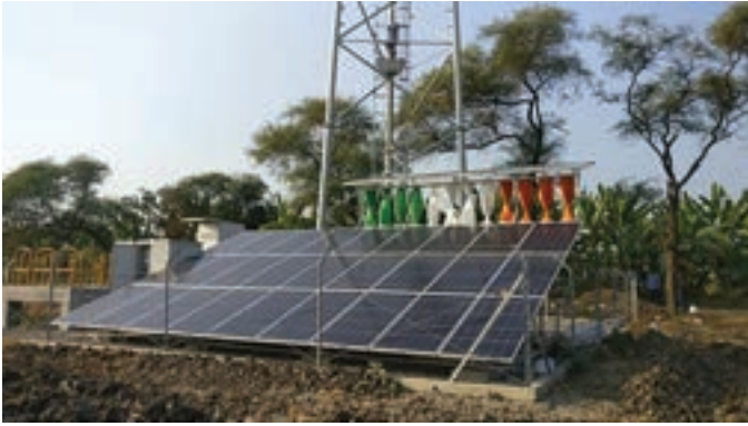
Figure 6: 11kW Installation for Telecom Tower
