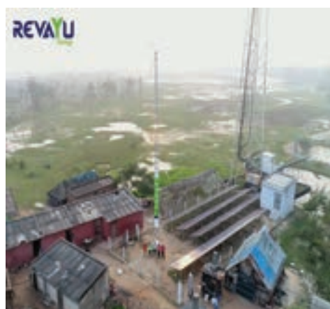
Figure 1: A Telecom Tower with Wind–Solar Hybrid Energy System
